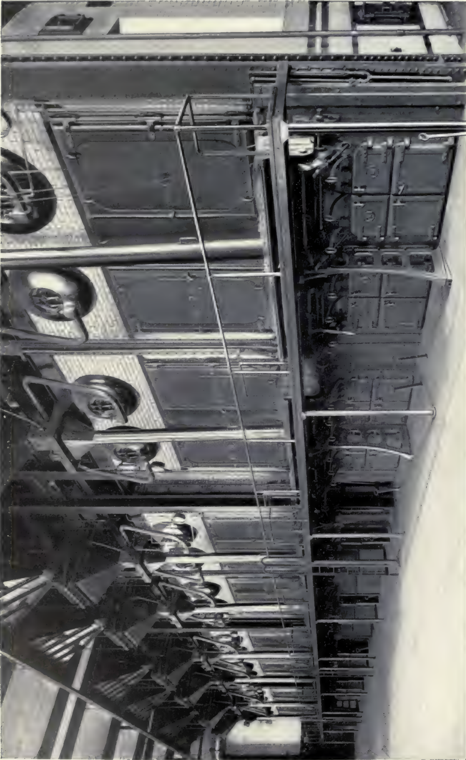
EDISON ELECTRIC ILLUMINATING CO., OF BOSTON, MASS. "L" STREET STATION. BABCOCK & WILCOX SUPERHEATERS INSTALLED IN 29,000 HORSE POWER OF BABCOCK & WILCOX BOILERS. THIS COMPANY OPERATES IN ITS VARIOUS STATIONS 39,000 HORSE POWER OF BABCOCK & WILCOX BOILERS AND SUPERHEATERS
